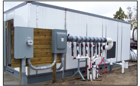
Remediation System designed by SESCO Engineers
